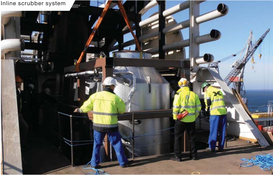
Inline scrubber system
